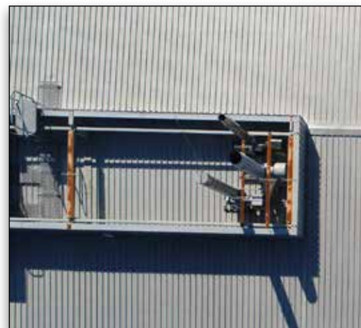
Skand projects AI-identified defects onto the ContextCapture reality mesh including forms of corrosion and building material degradation.
